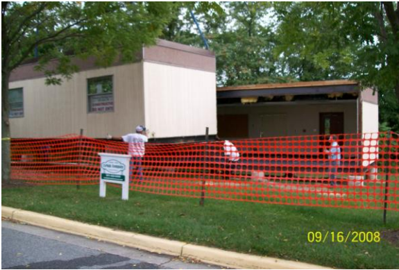
The back half is in place. Now the crane is moving the front half. The men are guiding it as it swings freely in the air.
