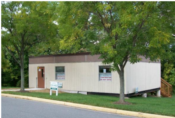
The outside of the building is almost complete. Skirting will be installed under the building and cosmetic work such as painting, shutters, and landscaping will finish the exterior.
