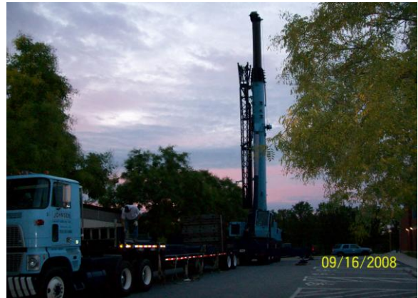
Finally the big day has come and the crane arrives at 6:30 AM to move the two halves of the museum on to the new foundation.
